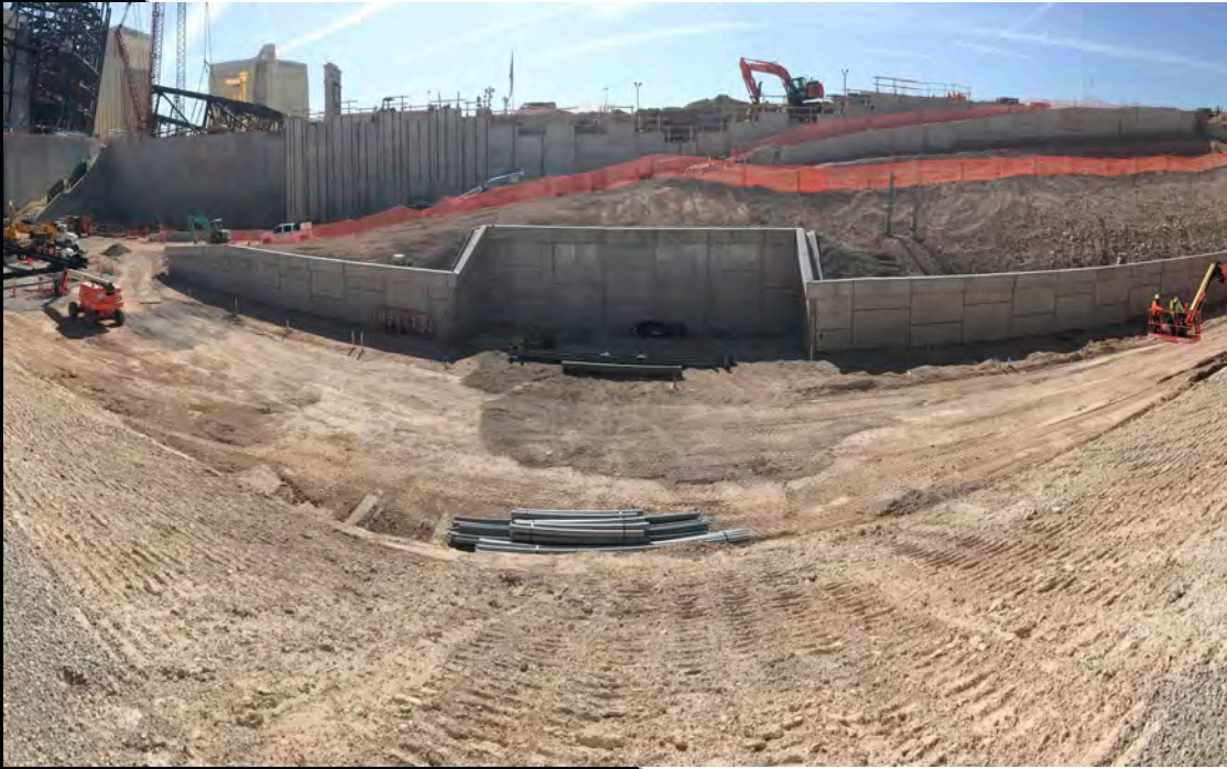
Above: East side field tray MSE wall installation progress. Below: Field tray rail grade beam preparation work under the south end longspan trusses.
